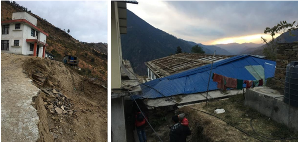
Figure 3: 8m deep open excavation adjacent to residential quarters (left) and Demolition of In-patient block (right)
