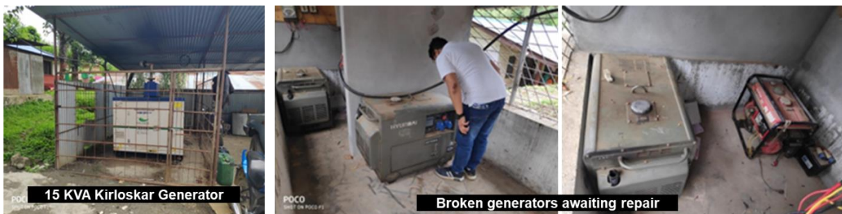
Figure 12: Generators at the hospital
