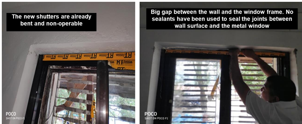
Figure 9: In-operable shutters and poor workmanship
