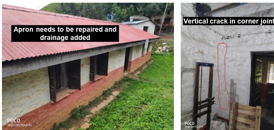
Figure 14: Defective aprons and corner cracks
