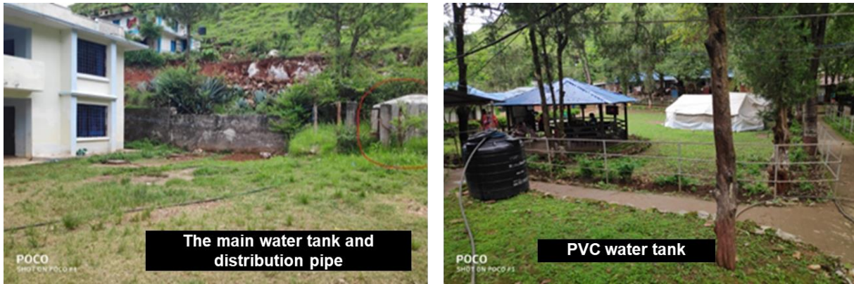
Figure 11: Water storage and distribution at the hospital
