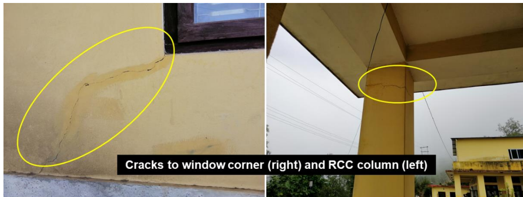
Figure 11: Settlement and /or seismic cracks
