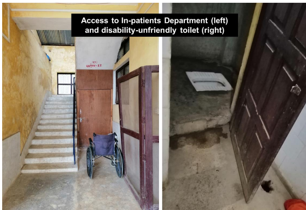
Figure 10: Access to In-patients Department and Step toilet limiting access for people with disabilities
