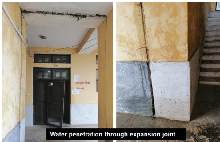
Figure 12: Water penetration through expansion joint
