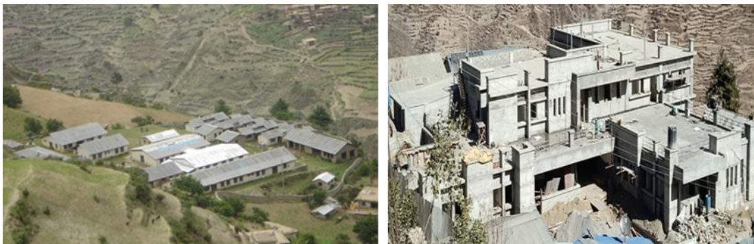
Figure 5: Mugu District Hospital – before upgrading (left) and current state of construction (right)
