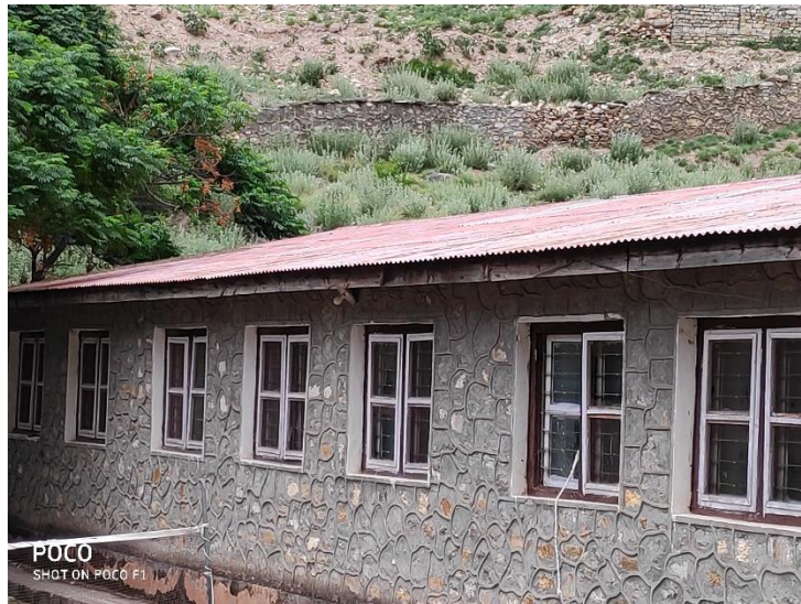
Figure 10: Building without seismic resilient elements - sills and lintels – at the windows
