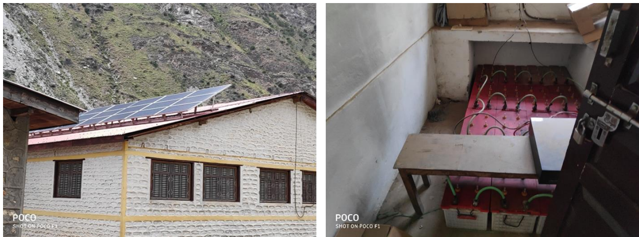
Figure 3 (left) Solar Panel on BEOC building (right) Solar Power Battery (not working) inside the BEOC building
