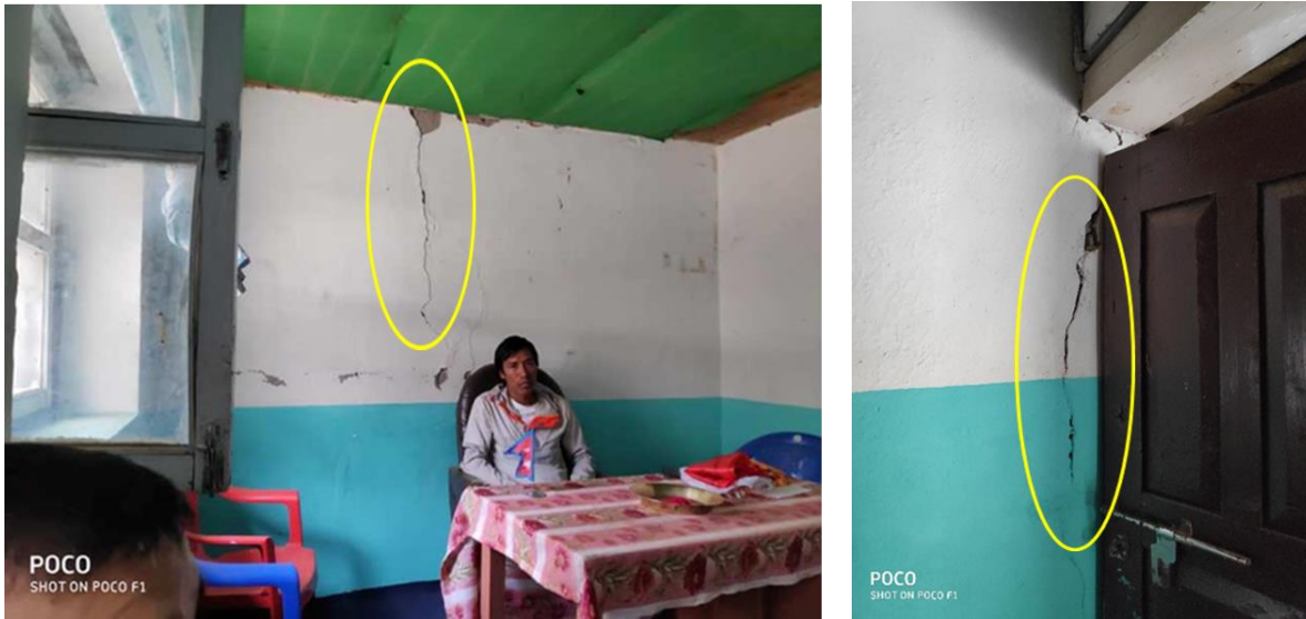
Figure 7: Cracks in the main building
