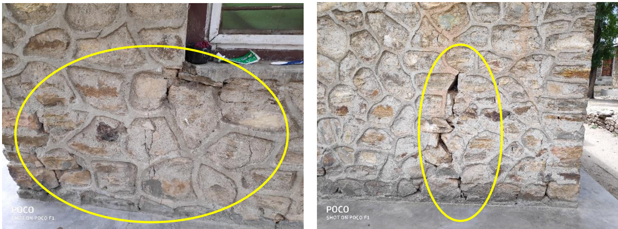
Figure 8: Cracks on the outer wall of the quarter
