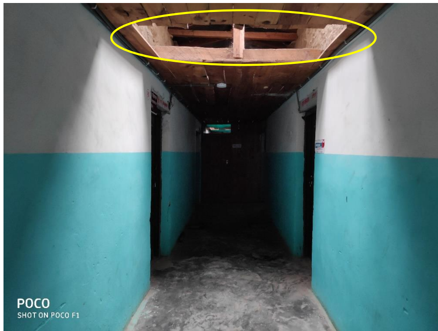
Figure 12. Unreinforced masonry wall above the false ceiling
