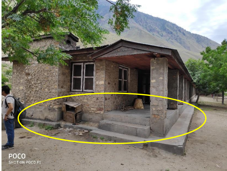
Figure 9: Lack of maintenance to stone and concrete elements
