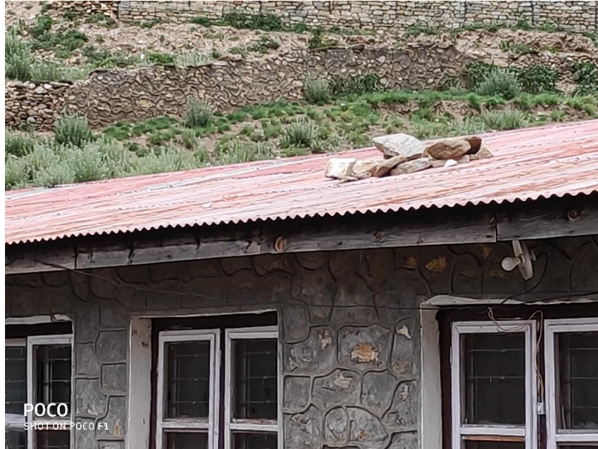
Figure 11: CGI roofing needs replacement and proper anchorage
