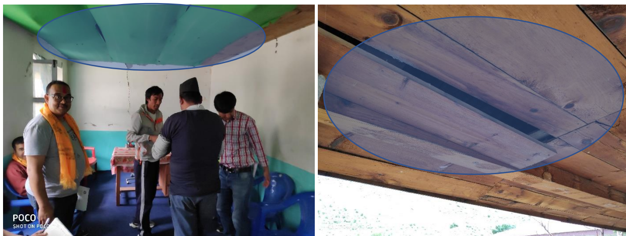
Figure 19: False ceilings requiring repair or replacement
