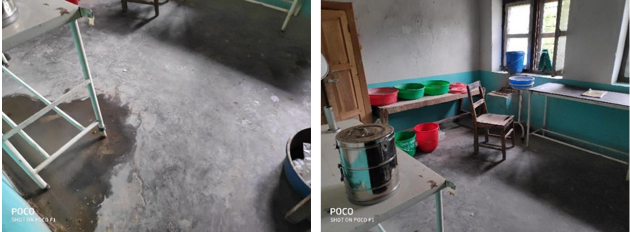
Figure 17: Interior floor finishes in poor condition
